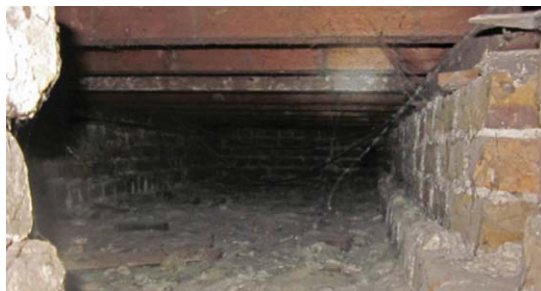
Figure 1. The floor before insulation by Q-Bot. (Photo courtesy of Matthew Holloway, Q-Bot MD.)
