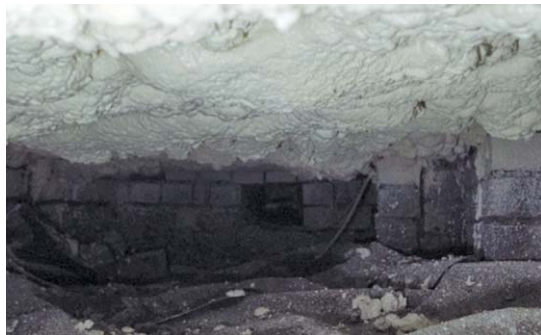
Figure 2. The floor after insulation by Q-Bot. (Photo courtesy of Matthew Holloway, Q-Bot MD.)
